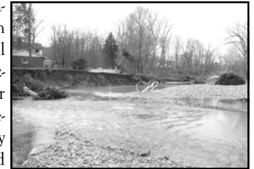
Gas pipeline and County Road jeopardized by erosion in the Town of Boston
